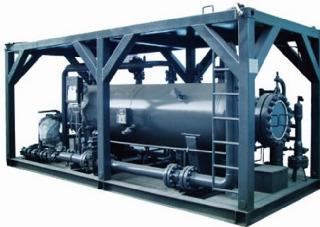
Fig. 3.8. Test separator unit at production site.
